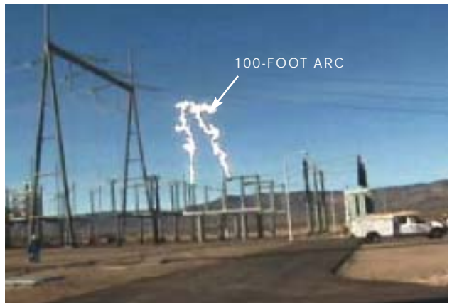
Figure 1 A switch failure at the Eldorado substation in Boulder City, NV, sent this 100-foot long, 500-kV arc into the air (courtesy Stoneridge Engineering, www.teslamania.com ).
