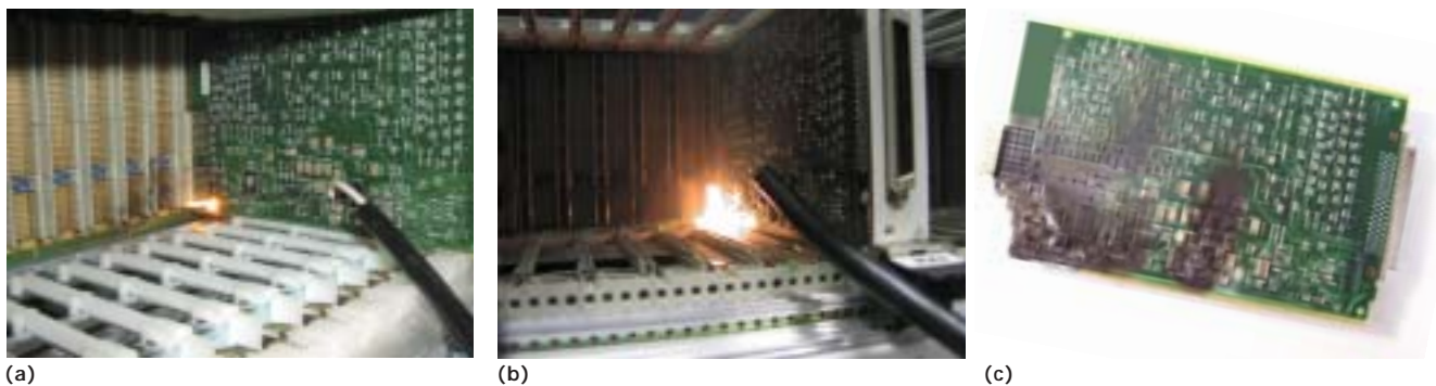
Figure 4 Without proper current limiting, a shorted capacitor in the 5V-dc circuit of a pc-board assembly can start a fire within seconds (a). After 30 sec, the fire has caused considerable damage (b), destroying the pc board and connector (c).
